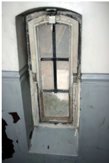
One of the small pivot windows in the corridor on the third floor corridor
