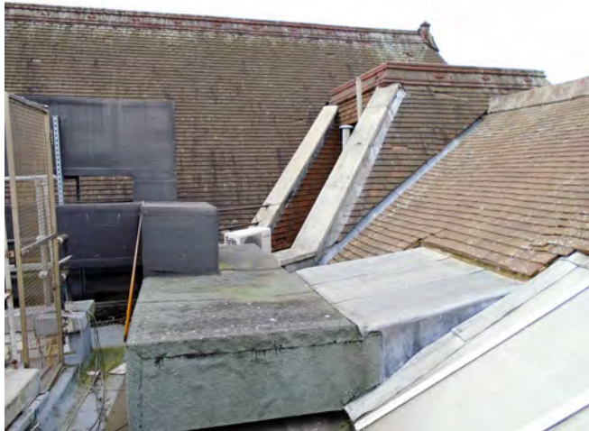
Duct work protruding through the roof fabric
