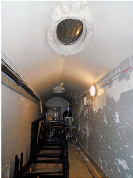
Linear corridor to the west of the concert hall is now being used as a storage area and is suffering from damp. The deterioration has caused for the paint finish to flake and detach, however, the moulded vent surround still remains intact.
