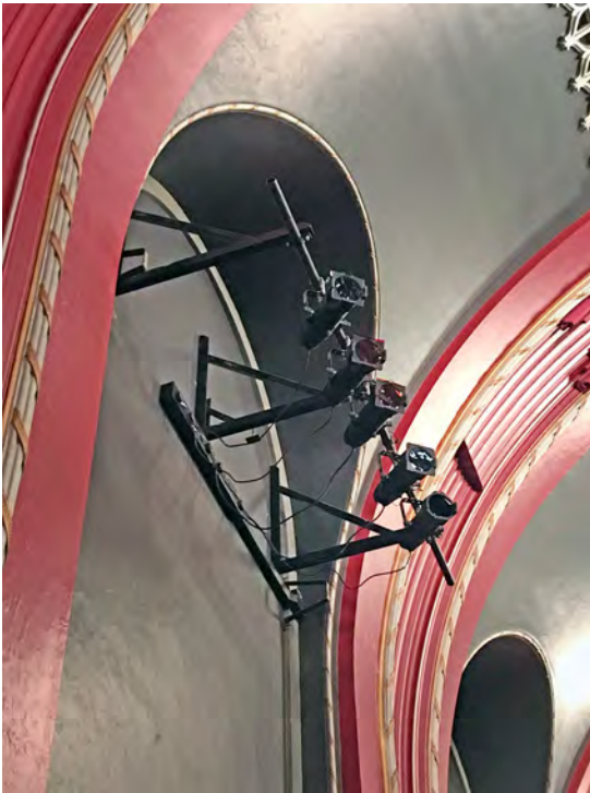
Wall fixed lighting brackets
