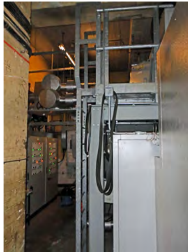
Basement electrical mechanical room
