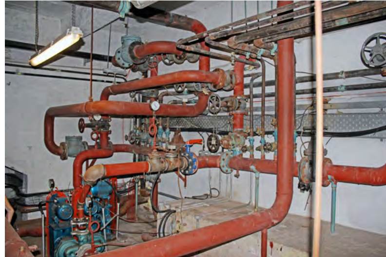
B2: Plant within the basement
