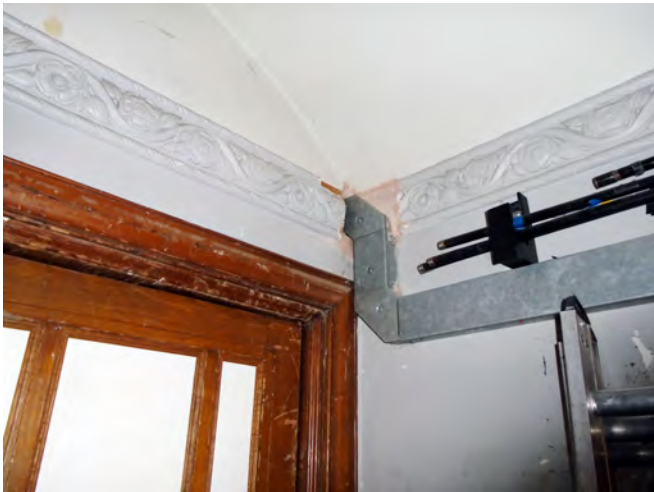
Service trays protruding through wall
