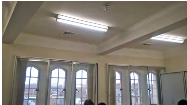
Typical office layout showing the downstands in the ceiling and the secondary glazing to the windows
