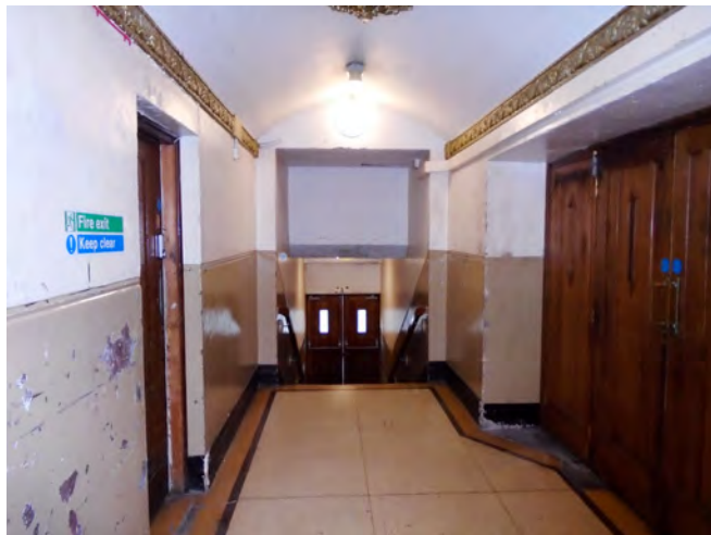
Back of house circulation spaces poorly kept with damage to wall and floor fabric
