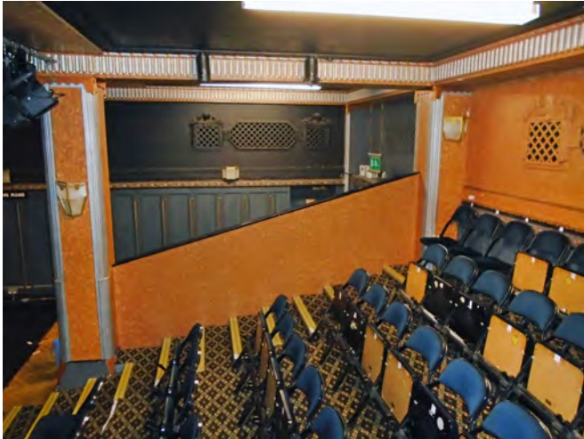
The seating in the studio, showing the later decorative features and sub-division
