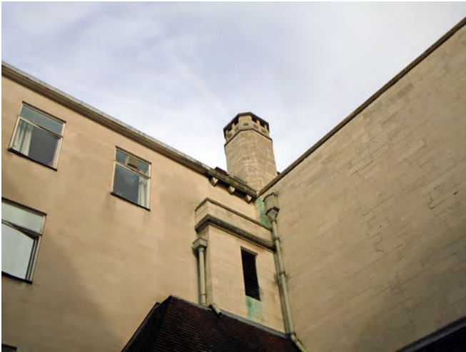
Existing west elevation of the Broadway Theatre at high level joining the neighbouring Civic Suite to the left-hand side
