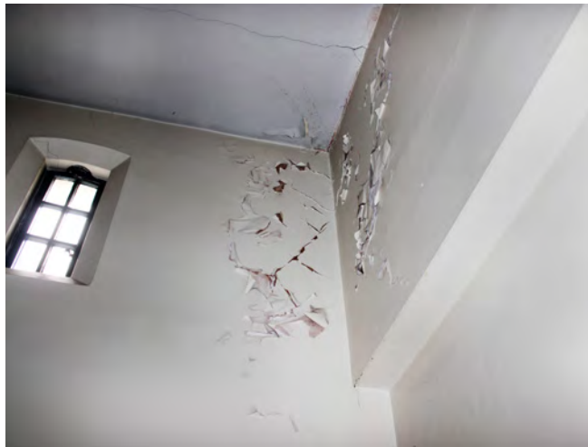
Areas of peeling paint within damp, poorly ventilated areas of the building
