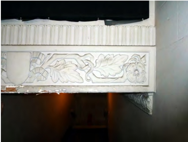
Detail of the high decorative moulded cornice within the secondary circulation spaces
