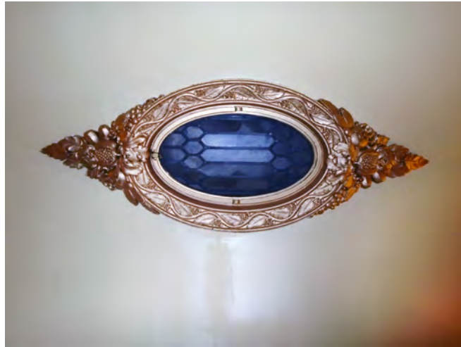
Moulded surround to the vent in the ceiling of the linear corridor to the east of the concert hall
